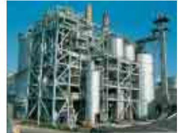
Fluidized bed boiler at the Kurashiki Plant (Tamashima)
