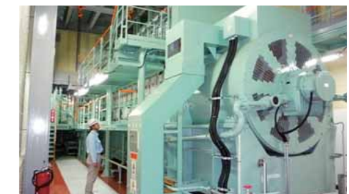
Gas engine power generation facility
